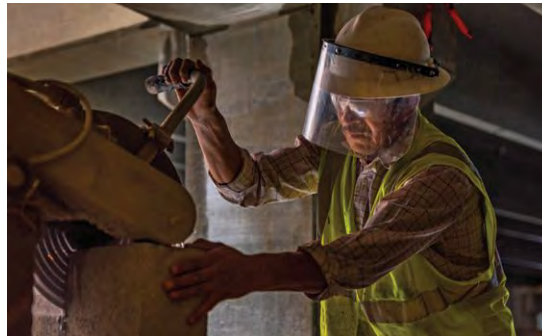
MASONRY A mason cuts materials for the 6th-floor corridors and parking garage vestibules.
