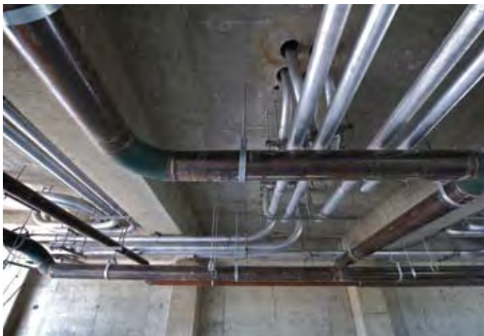
Under slab piping and conduit at new generator building
