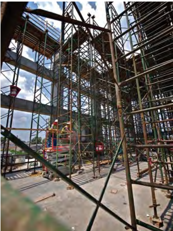
Operating floor of generator building
