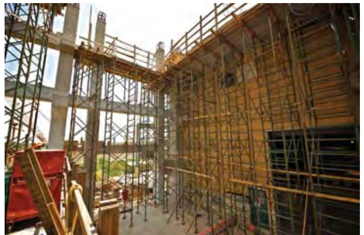
Loading bay connects existing pump station to new generator building
