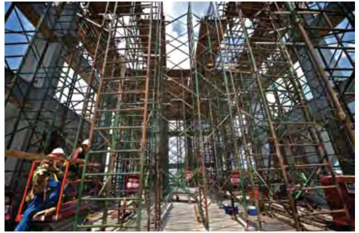
Operating floor of generator building
