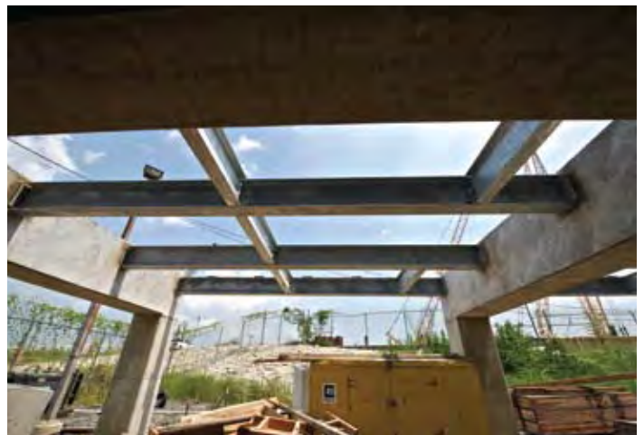
Radiator and day tank platform
