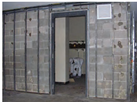
Restoration took place in phases with hundreds of workers and contractors involved in the major construction efforts.
