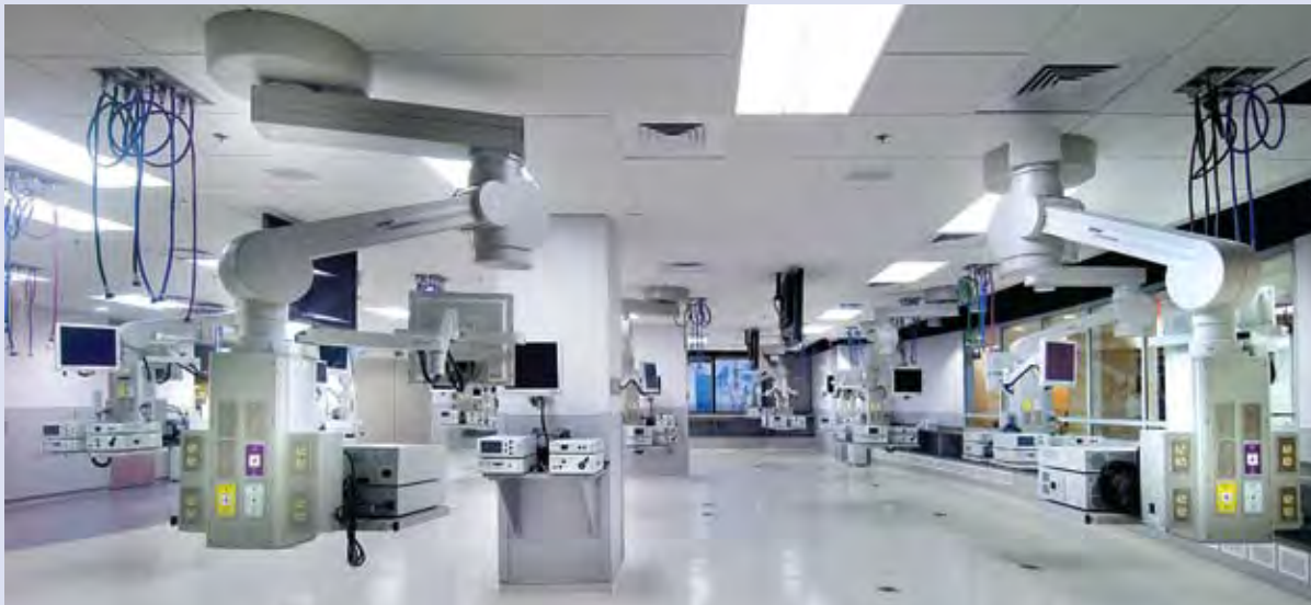
Restructuring of the LSU School of Medicine training lab involved extensive rough-in construction above the ceiling height to carry HVAC ductwork, cables, medical gases tubulars, electronic media, and other equipment in the overhead space. The McDonnell Group completed demolition, construction, and medical equipment installation on a tight schedule.
